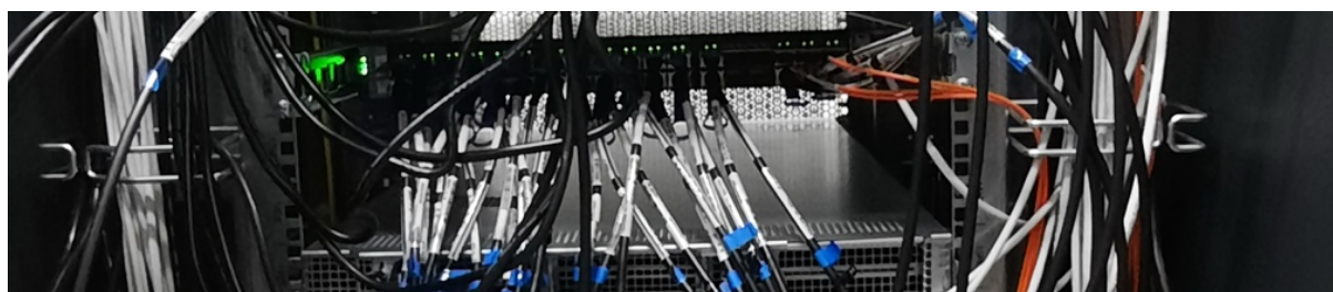
Infiniband networks need short cables and connect at the back of the switches
