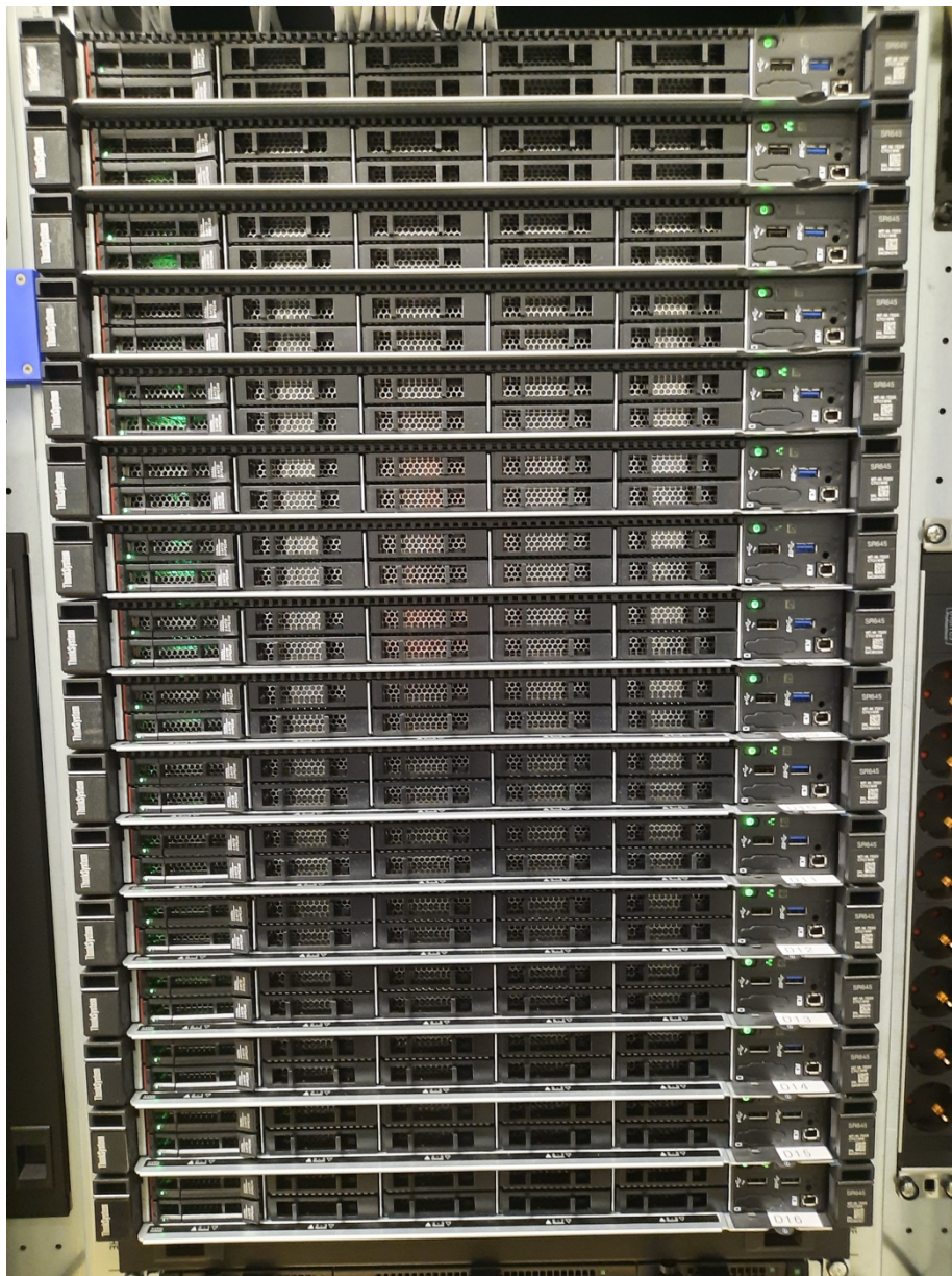
Compute nodes as these node-d systems send operational data to the monitoring servers, which trigger alerts in case of problems
